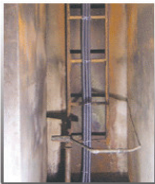
Cable mounted for fire test
